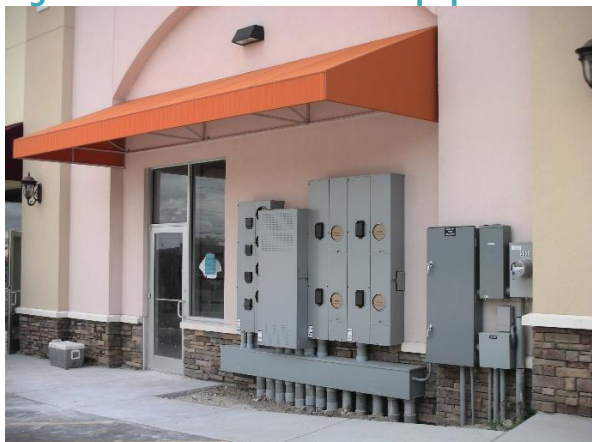
Prohibited (utilities facing street)
