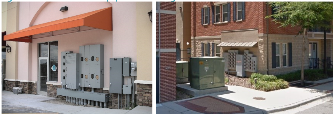
Prohibited (utilities facing street)
