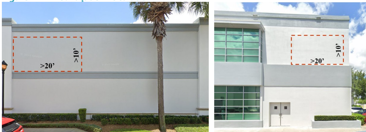
Examples of blank wall exceeding 20 horizontal feet by 10 vertical feet without articulation
